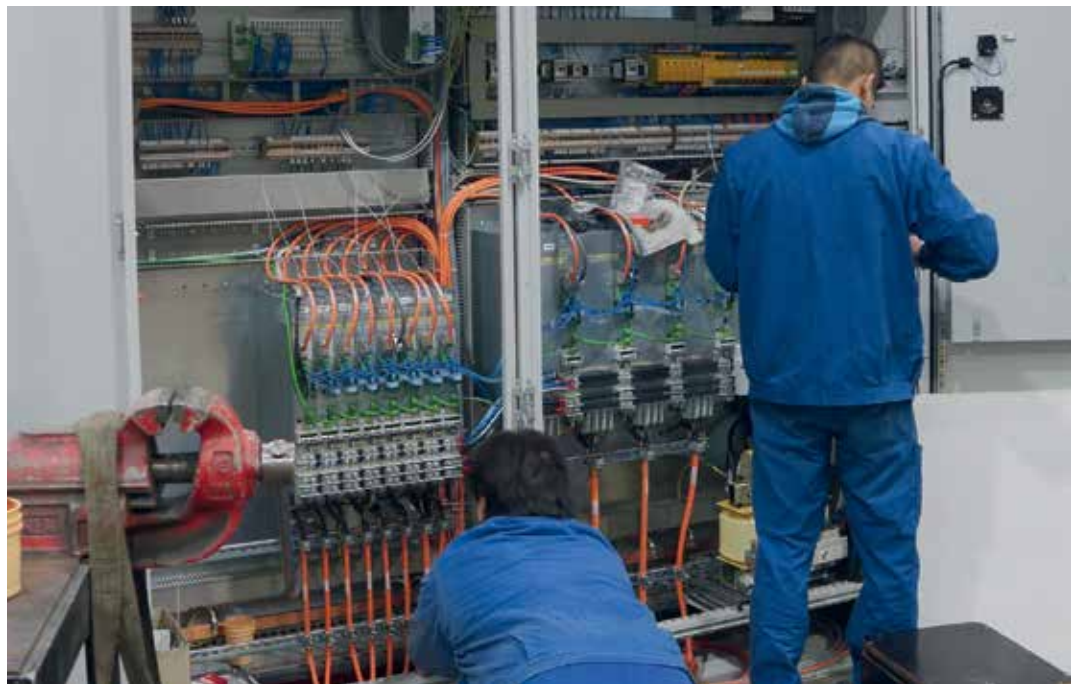
Hydraulic and electrical installations as well as the entire machine safety system are newly installed during a general overhaul. This is due to the fact that statutory safety regulations have usually changed since the machine was first put into operation.
