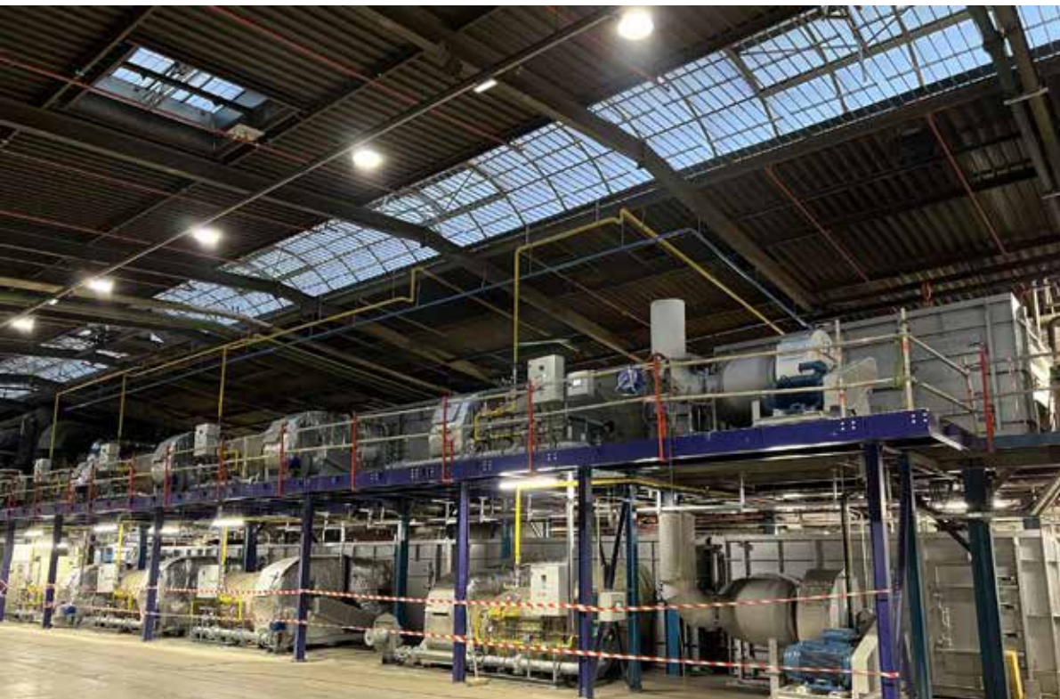
Curing ovens at Arconic coil coating line
